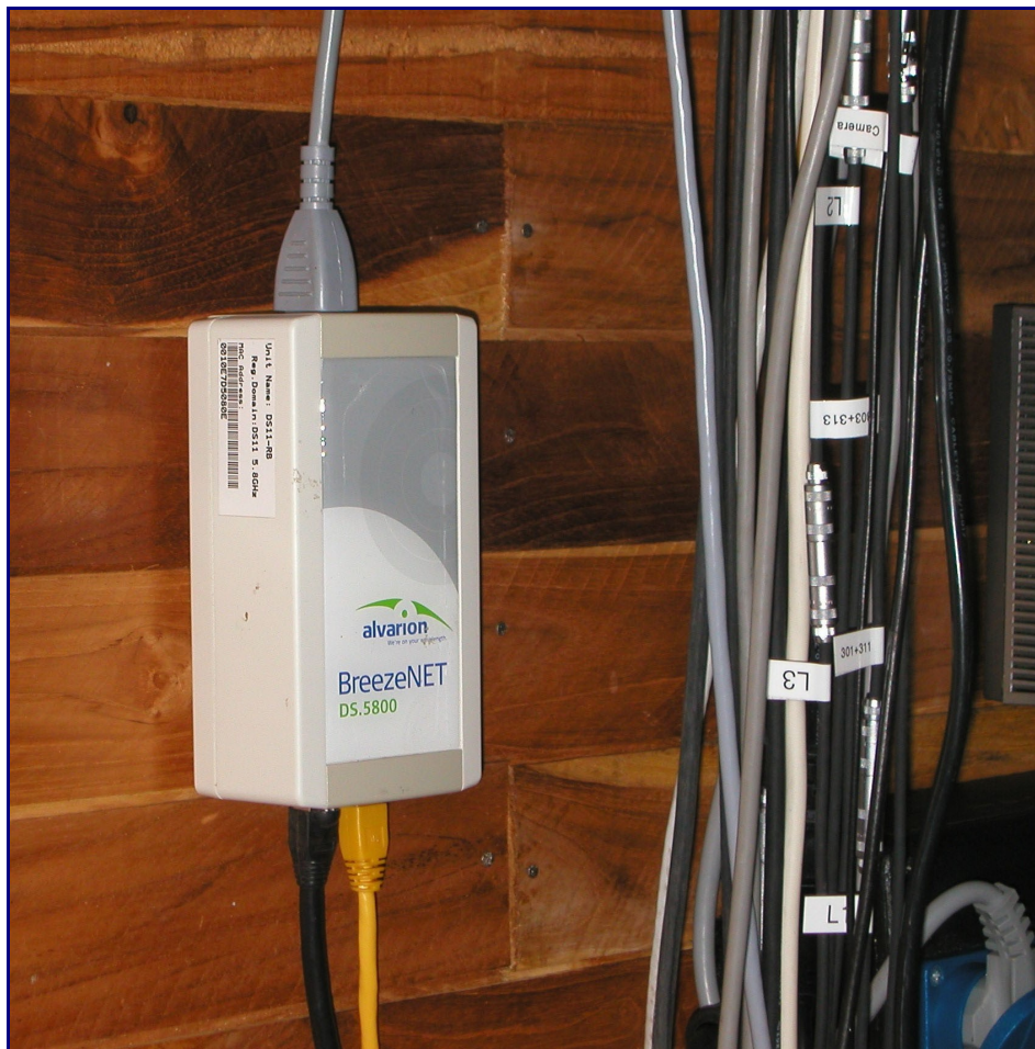
Figure 6: Alvarion DS5800 IDU installed in Pico Espejo.
