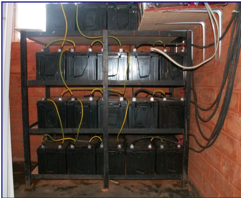
Figure 9: A battery bank of 3600 Ah, currents reach levels of 45 A during charging
