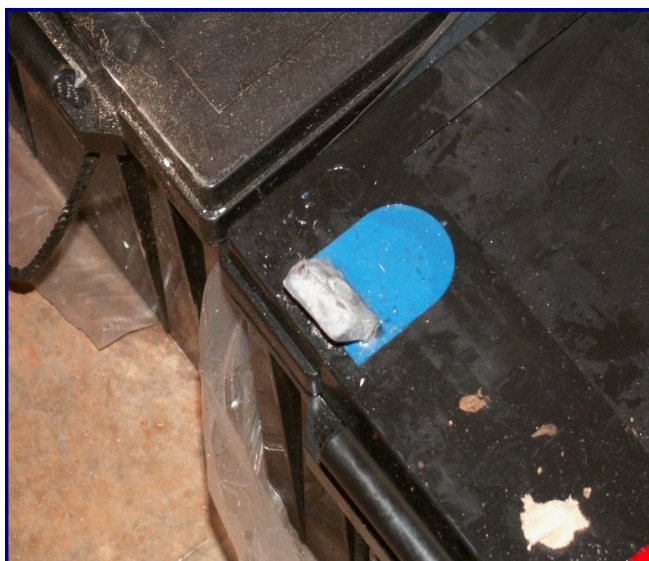
Figure 3: Lead-Acid 200 Ah battery. Detail of the effect of the weight on the terminals during transportation
